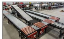
24-Volt Conveyor & Zone Routing
